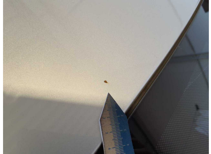
Damage 10: Roof: Roof - Corrosion - Repair and paint
