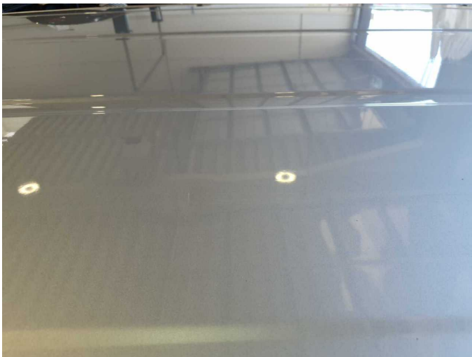
Damage 10: Roof: Roof - Corrosion - Repair and paint
