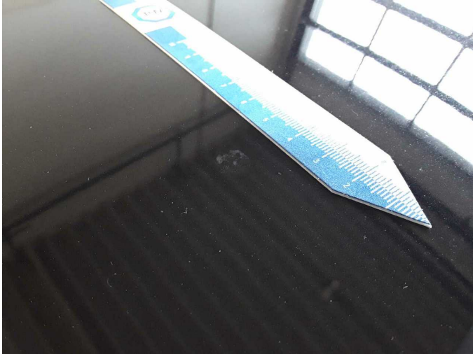
Damage 8: Roof: Roof (Anätzung) - Paint defect - Repair and paint
