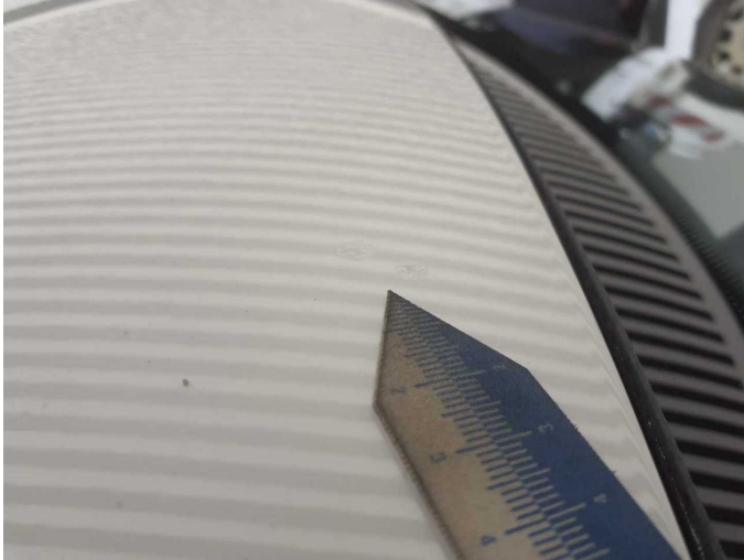
Wear and tear 4: Roof: Roof (Lack stiff) - Paint defect - No deduction
