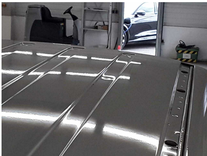
Damage 8: Roof: Roof - dent(s) - Smart repair
