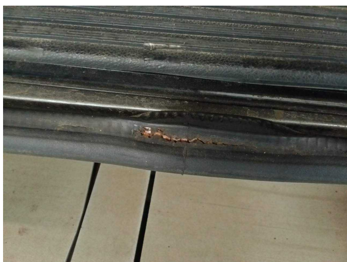
Damage 6: Sliding door, right: Door seal - Damaged - Replace
