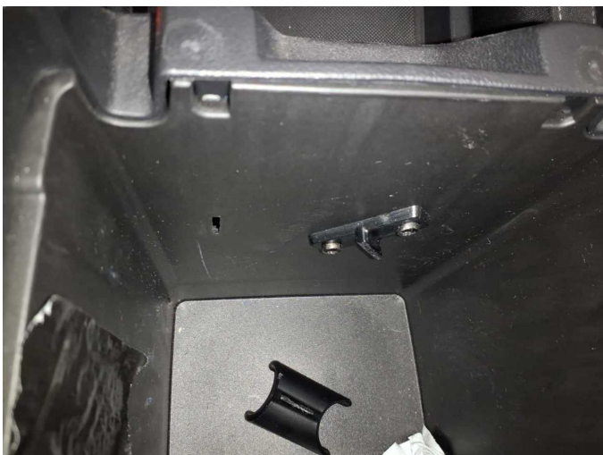
Damage 6: Interior: Arm rest, front (Deckel hinten, Fehlbohrungen) - Differs from the original configuration - Replace
