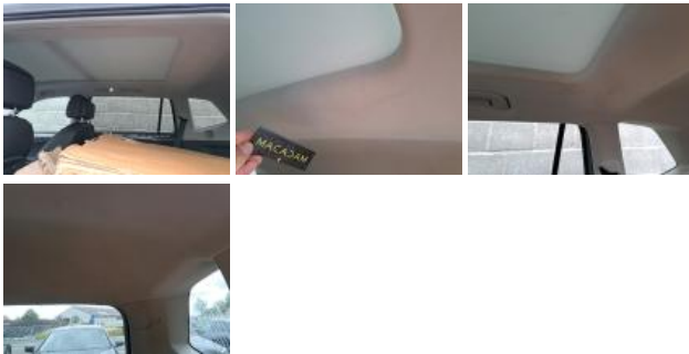
Interior covering A pillar R, Scratch(es), Acceptable
