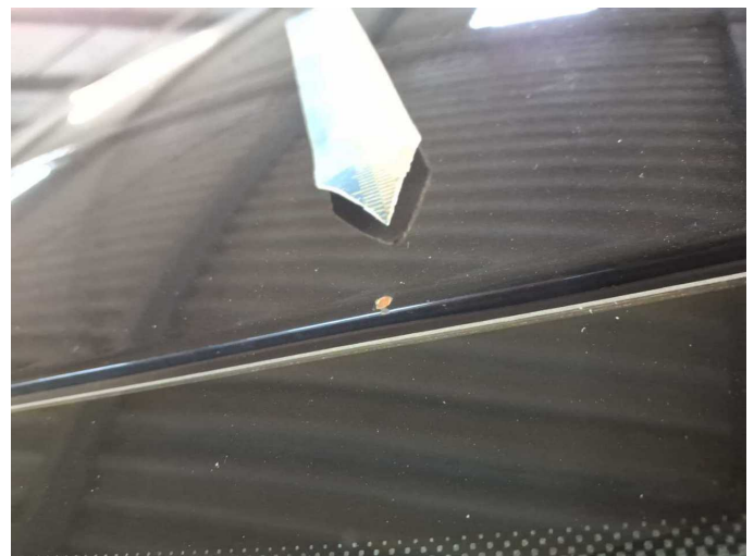
Damage 11: Roof: Roof - Corrosion - Repair and paint
