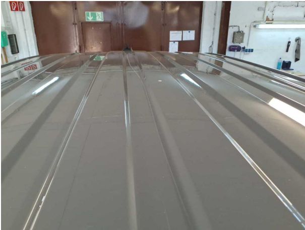
Damage #1: Roof: Roof - Scratched - Cover / polish
