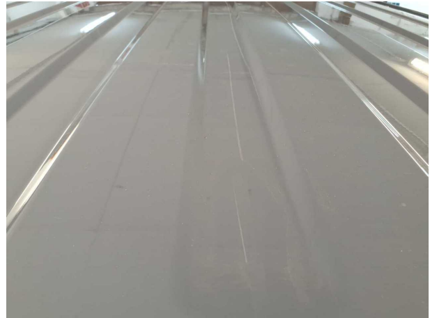
Damage #1: Roof: Roof - Scratched - Cover / polish
