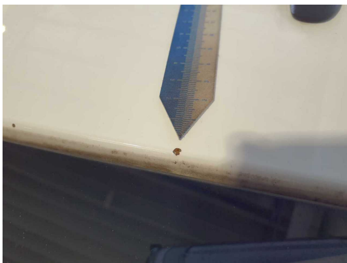
Damage 4: Roof: Roof (Dachkante) - Corrosion - Paint
