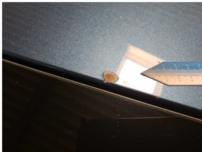
Damage 17: Roof: Roof - Corrosion - Smart repair
