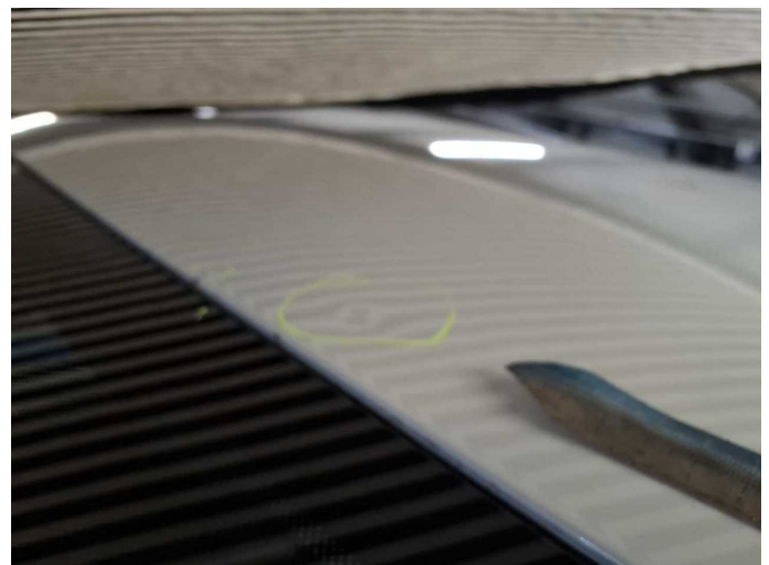
Damage 8: Roof: Roof - Dent / paintcoat damage - Repair and paint
