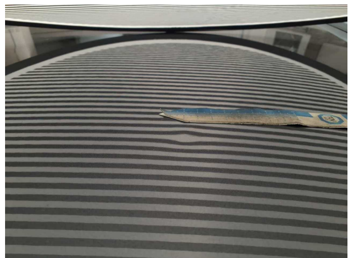
Damage 5: Roof: Roof - dent(s) - Smooth repair work
