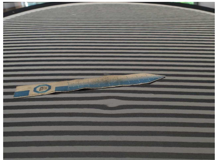
Damage 5: Roof: Roof - dent(s) - Smooth repair work
