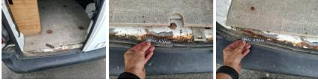
Bumper R, Deformed / Strained, Replace
