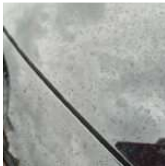
Damage Type Stonechipping
