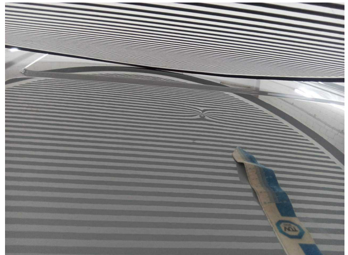
Damage 6: Roof: Roof - Dent / paintcoat damage - Repair and paint
