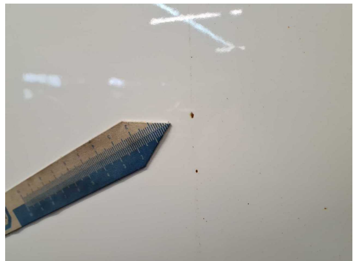
Damage 11: Sliding door - left side: Sliding door (Korrosion) - Scratched - Repair and paint
