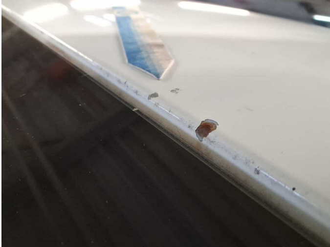
Damage 10: Roof: Roof (Korrosion) - Stone chips - Paint
