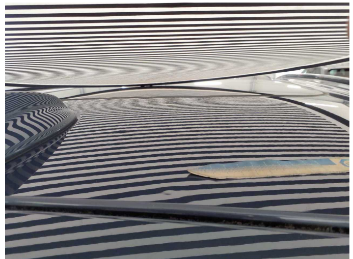
Damage 3: Roof: Roof - dent(s) - Smart repair
