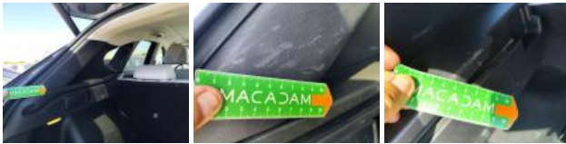
Rear roof pillar covering R, Scratch(es), Replace
