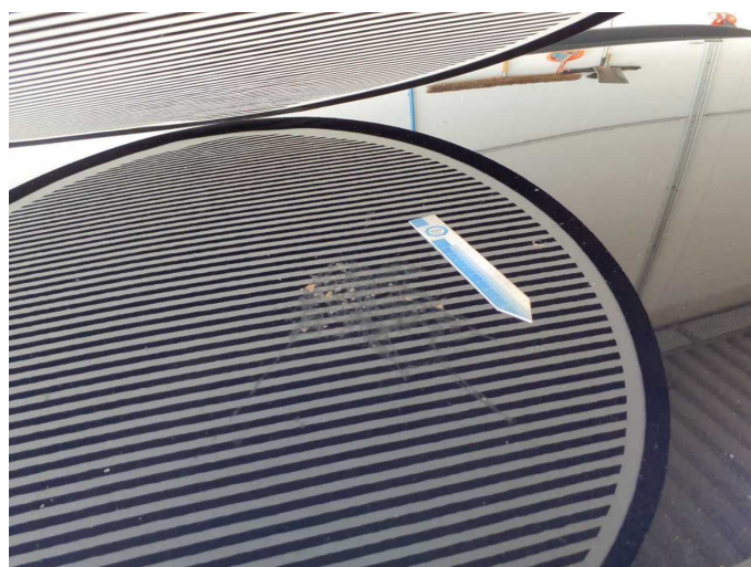
Damage 9: Roof: Roof (Anätzung) - Paint defect - Repair and paint
