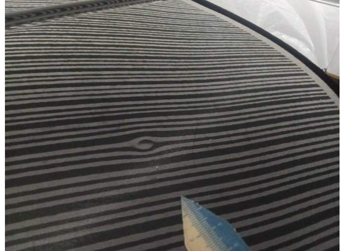
Damage 3: Roof: Roof - dent(s) - Smooth repair work
