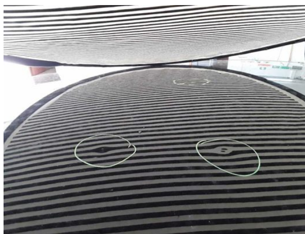
Damage #10: Roof: Roof - dent(s) - Smooth repair work
