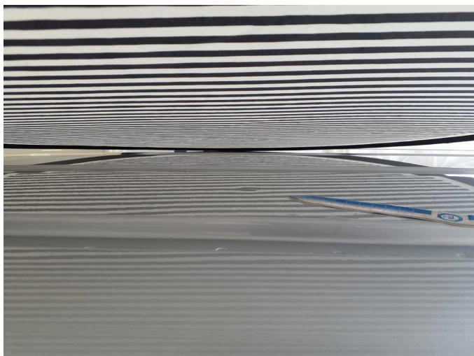
Damage 5: Roof: Roof - dent(s) - Smooth repair work
