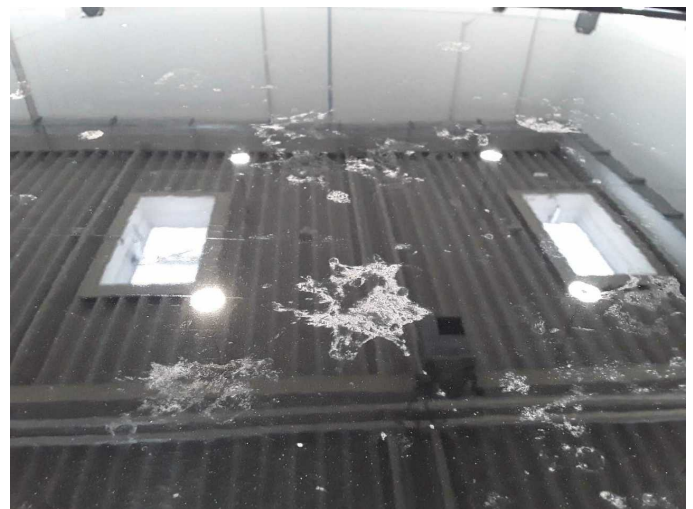
Damage 7: Roof: Roof (Anätzung) - Paint defect - Repair and paint
