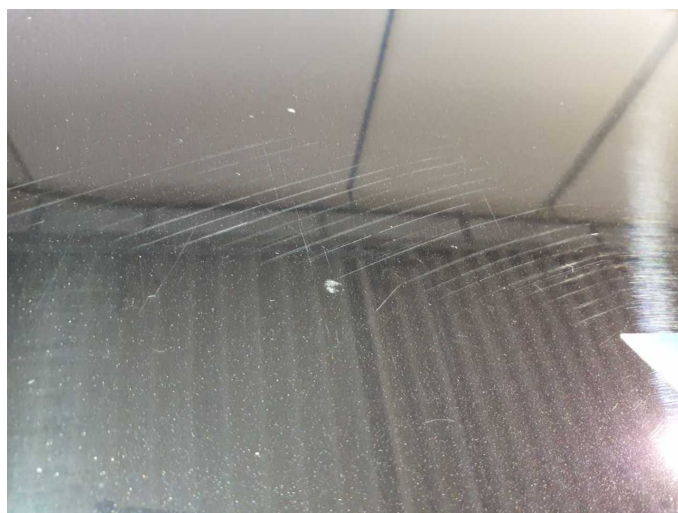
Damage 17: Roof: Roof - Scratch(es) - Paint
