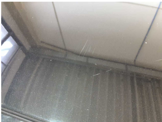
Damage 17: Roof: Roof - Scratch(es) - Paint
