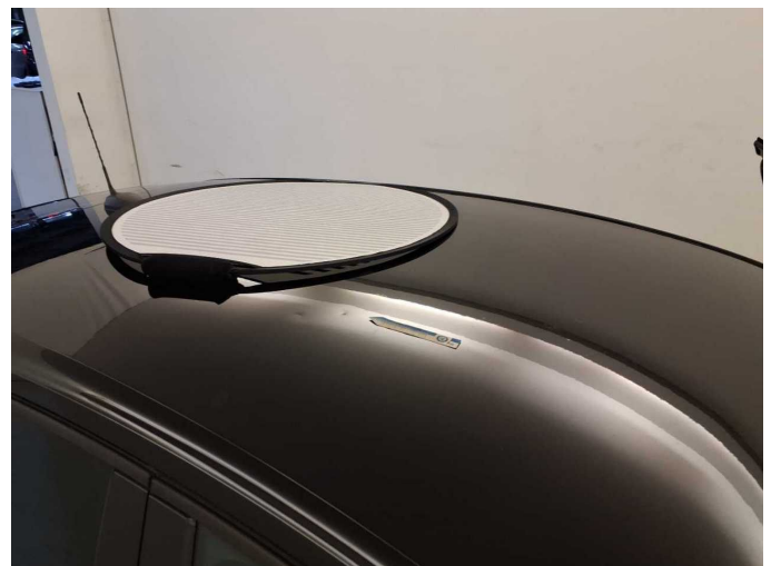
Damage 9: Roof: Roof - dent(s) - Smooth repair work
