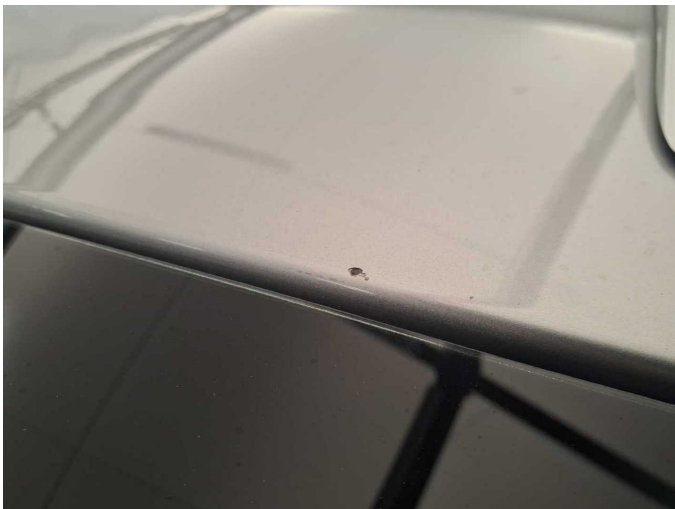
Damage 1: Roof: Roof - Stone chips - Smart repair
