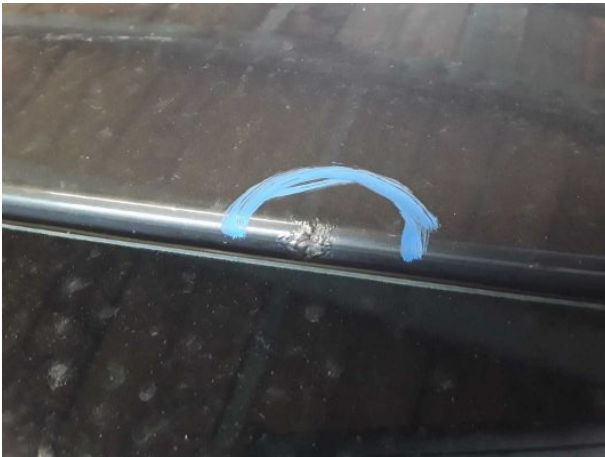
Damage #10: Roof: Roof - Corrosion - Repair and paint
