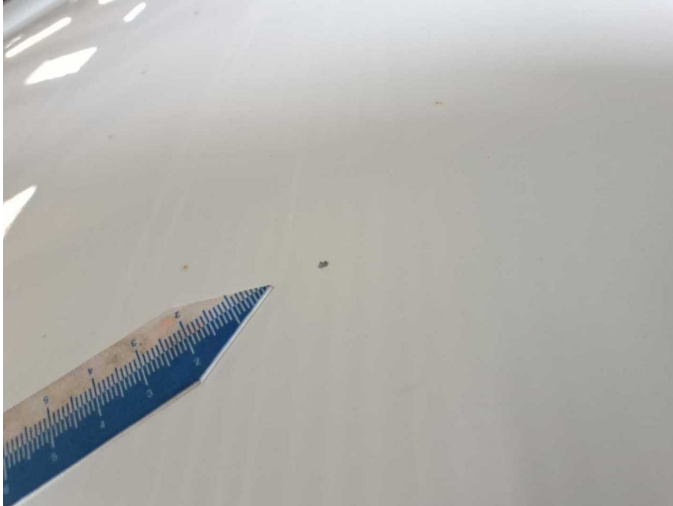
Damage 15: Roof: Roof - Stone chips - Paint
