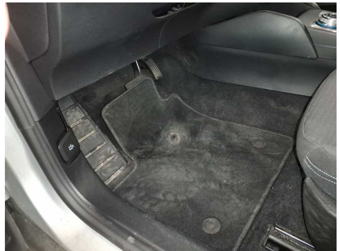
Damage 1: Trim / covers: Floor mats - Holes - Replace
