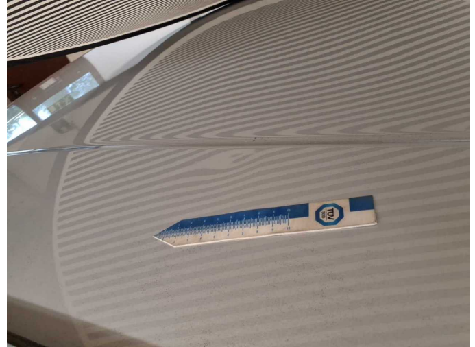
Damage 5: Roof: Roof - dent(s) - Smooth repair work
