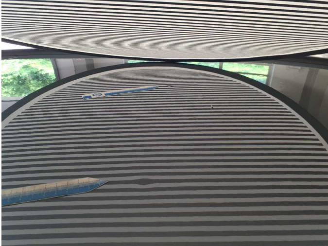
Damage 5: Roof: Roof - dent(s) - Smooth repair work
