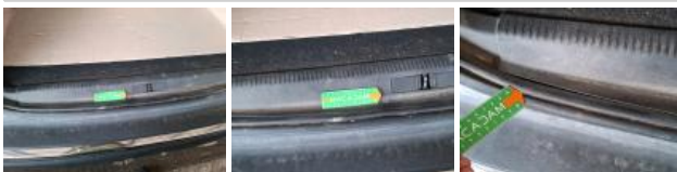
Boot lid covering R, Scratch(es), Replace
