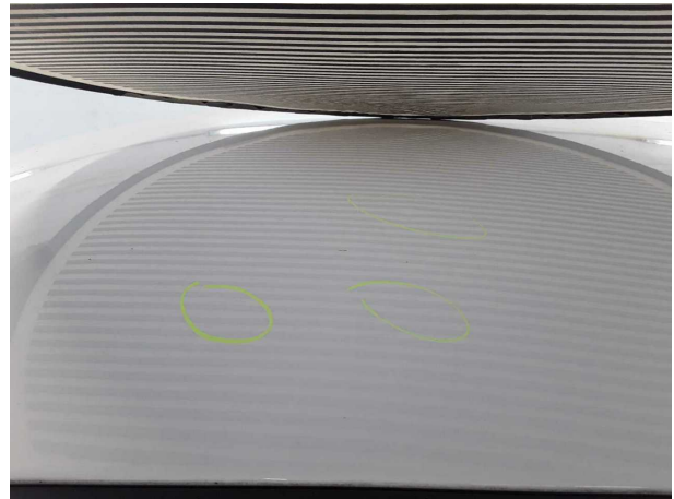
Damage #4: Roof: Roof - dent(s) - Smooth repair work
