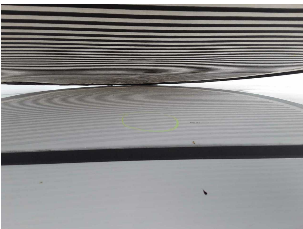
Damage #4: Roof: Roof - dent(s) - Smooth repair work
