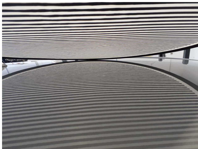
Damage 4: Roof: Roof - dent(s) - Smooth repair work
