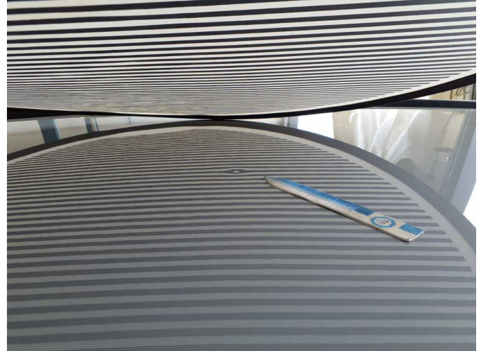
Wear and tear 7: Roof: Roof - dent(s) - No deduction
