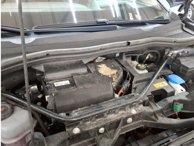
Damage 1: Air-conditioning system: Air-conditioning system (Isolierung Klimagehäuse) - Damage caused by marten / rodent - Replace
