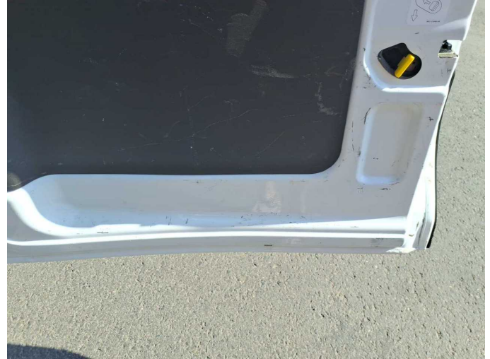
Damage 3: Boot lid / rear door: Rear door - right side (Innenseite) - Scratched - Smart repair
