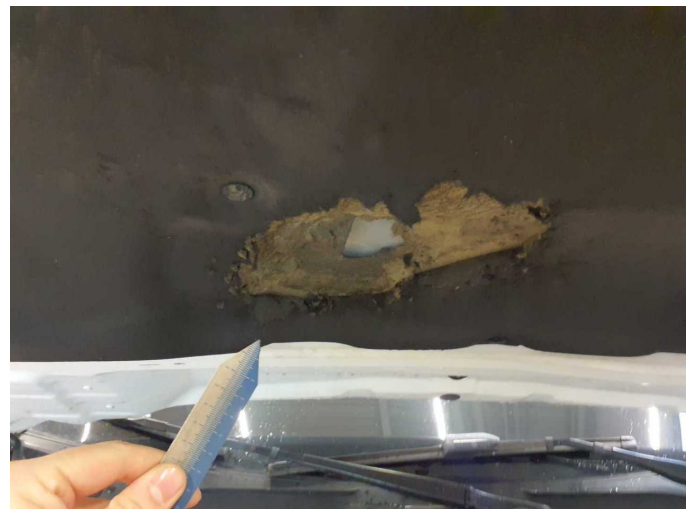
Damage 5: Bonnet: Insulation lining - Broken / torn - Replace
