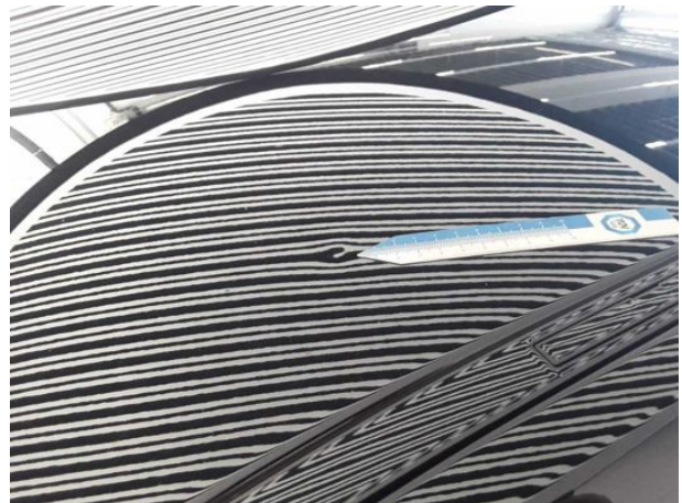
Damage #2: Roof: Roof - dent(s) - Smooth repair work
