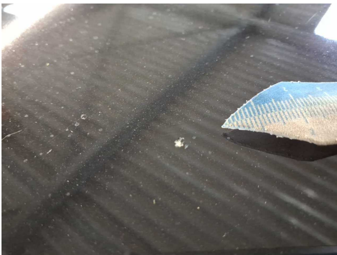
Damage 16: Roof: Roof - dent(s) - Smooth repair work
