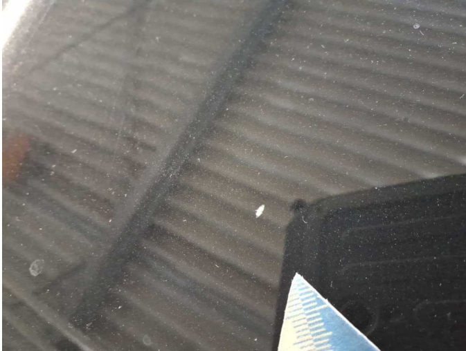
Damage 16: Roof: Roof - dent(s) - Smooth repair work
