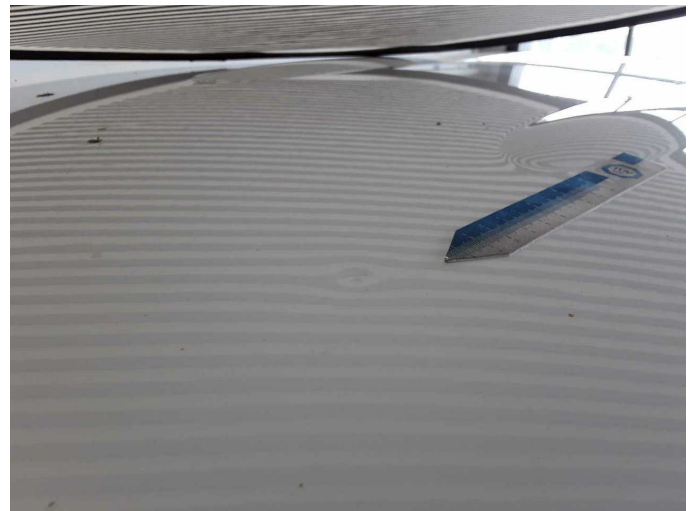
Damage 2: Roof: Roof - dent(s) - Smooth repair work
