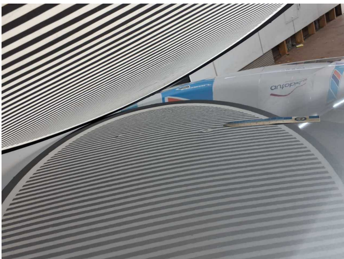
Damage 3: Roof: Roof - dent(s) - Smart repair
