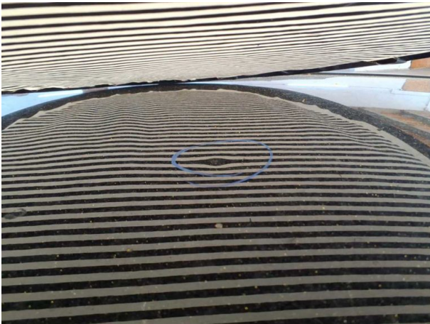
Damage #8: Roof: Roof - dent(s) - Smooth repair work
