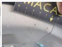
Engine insulation, Damaged, Replace
