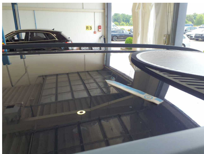
Damage 13: Roof: Roof - Paint defect - Repair and paint
