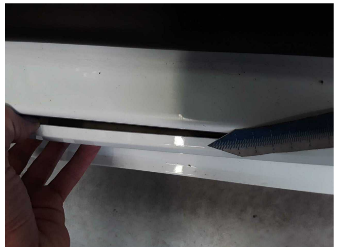
Damage 6: Sill - left side: Trim - Damaged - Replace
