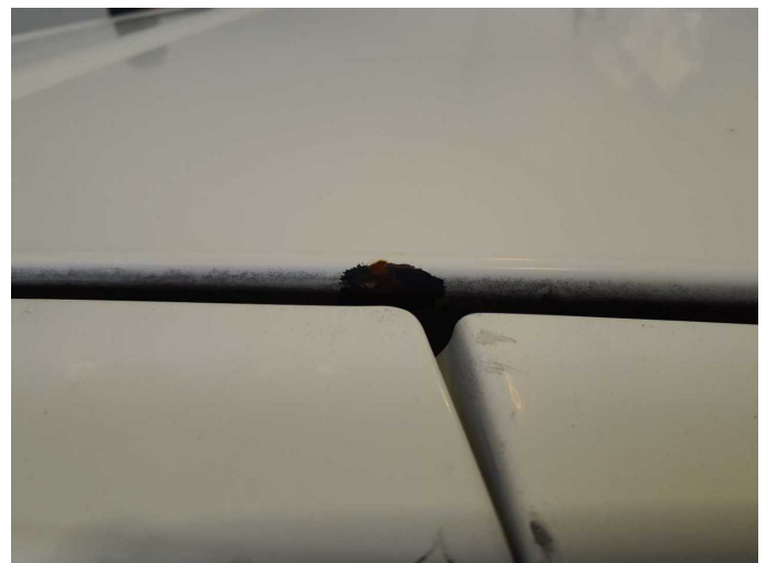
Damage 14: Roof: Roof - Corrosion - Repair and paint
