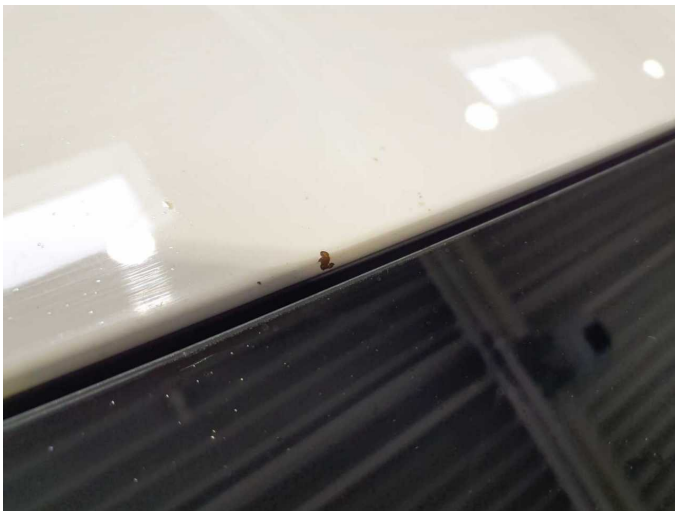
Damage 9: Roof: Roof - Corrosion - Repair and paint
