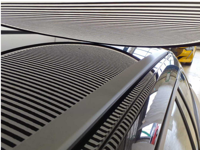
Damage 10: Roof: Roof - Corrosion - Repair and paint
