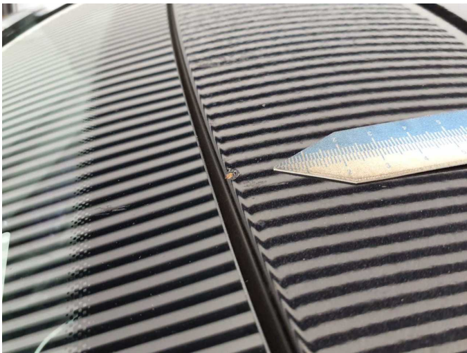
Damage 10: Roof: Roof - Corrosion - Repair and paint
