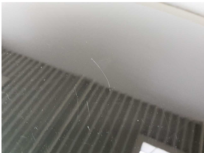
Damage 14: Roof: Roof - Scratch(es) - Paint
